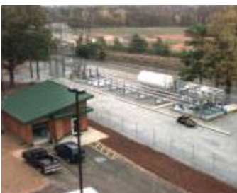
Southwire cable test site in Carrollton, Georgia
